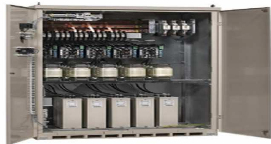
Figure 4. Three phase series reactors
