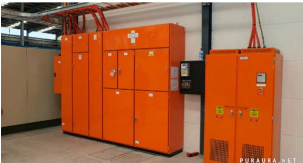
Figure 9. Automatic power factor correction unit separate from main switchboard.
